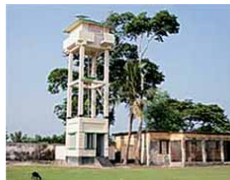
Figure 3: Water tank (Source: BRAC)
