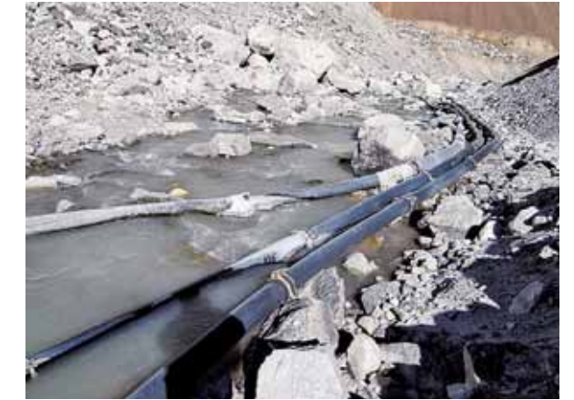
Figure 2: Pipelines to siphon water
