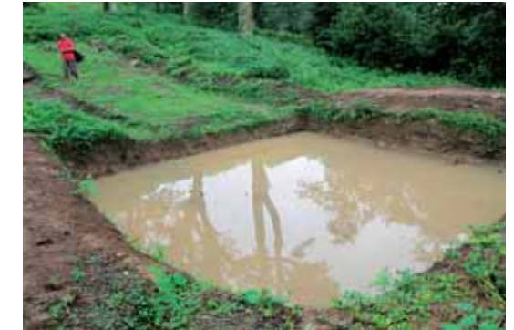
Image 2: Digging of ponds and lakes in the recharge areas helps to trap the surface runoff and supplement the natural ground water recharge
