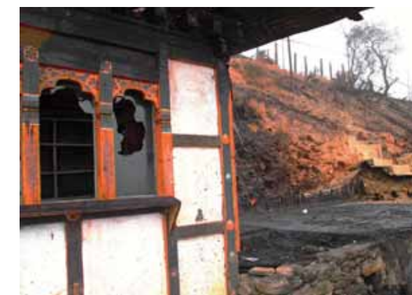
Figure 2: Premise destroyed by fire
